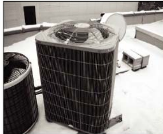
Air conditioning systems
