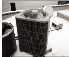
Air conditioning systems
