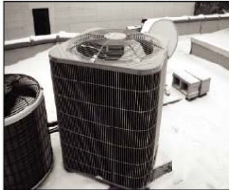
Air conditioning systems
